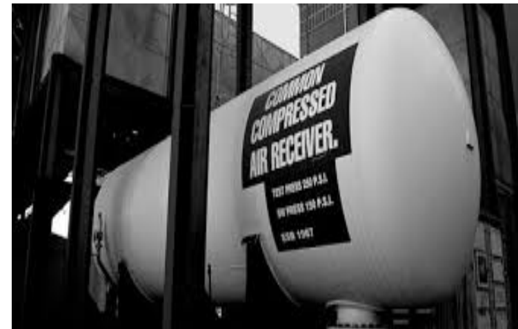
Compressed Air Energy Storage
