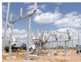
Goodwell Wind Substation
