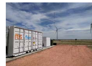
1.0MW/1.0MWh NREL Research Energy Storage
