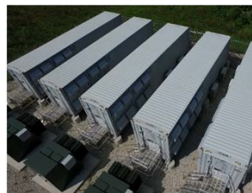
19.8MW/7.9MWh Jake Energy Storage
